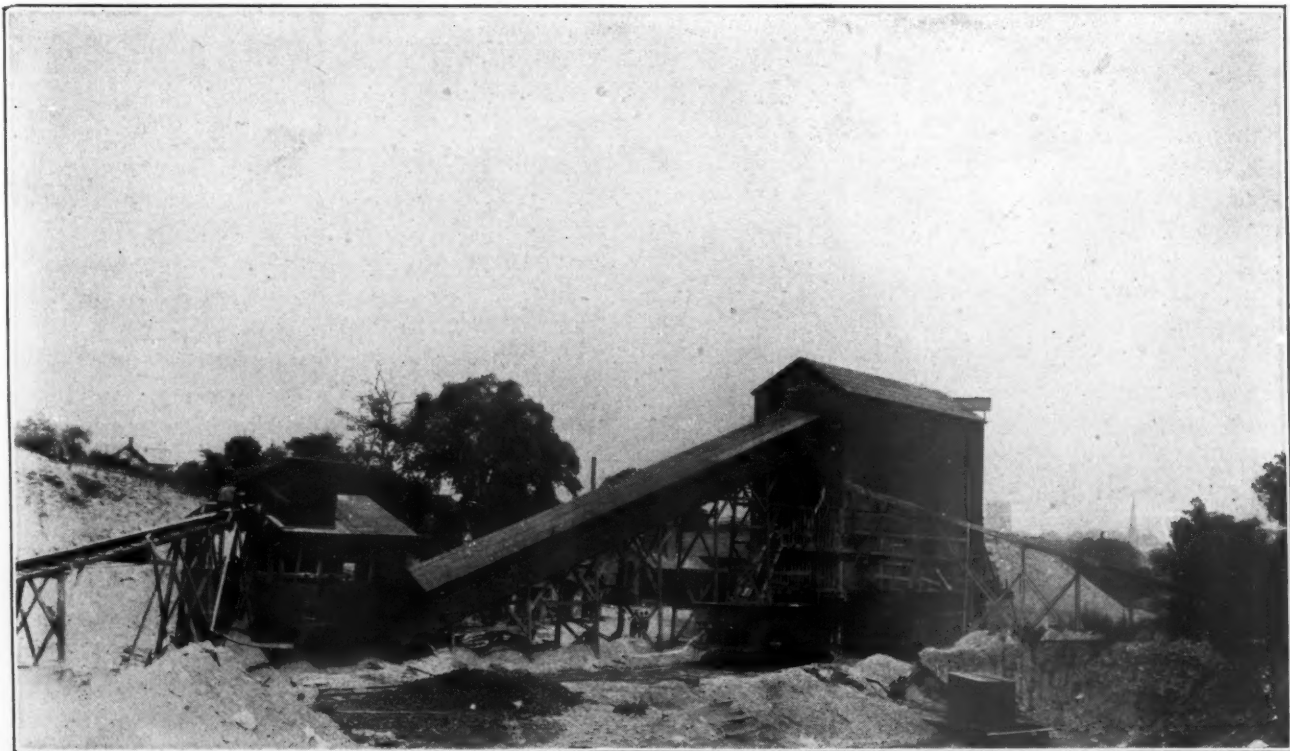
Screening and Crusting Plant at Left; Sizing and Bins at Right
